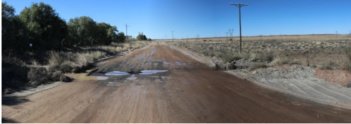
Figure 5: Gravel roads along the eastern and southern borders of the site will also result in localised transformation. Note how this road also influences the natural runoff patterns as it forms an obstruction to flow.
